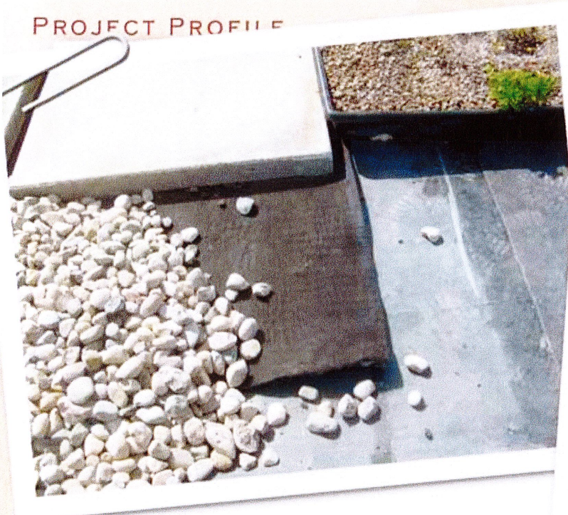
Shown are the construction material layers: waterproofing membrane, drainage and water retention mat, and green roof tray. Pavers and ballast are used in the nongreen areas.
