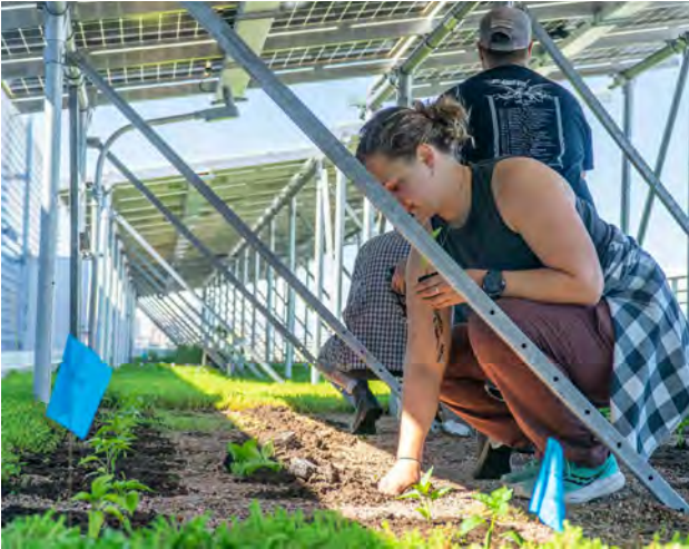
Setting up rooftop agrivoltaics under a solar PV array Credit: Kevin Samuelson, Colorado State University Spur
