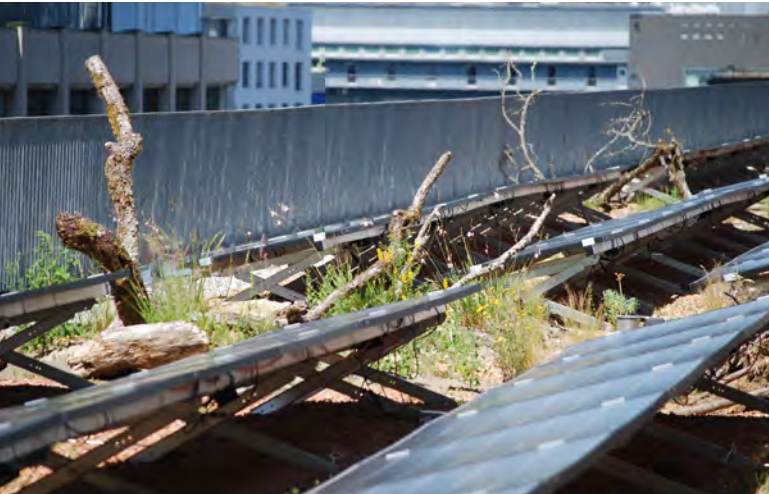
Biosolar green roof, Switzerland Credit: Elisabeth Weiss-Tessbach
