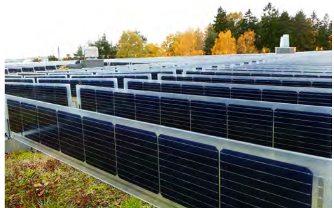
Office building, Oslo (Norway) Credit: Over Easy Solar
