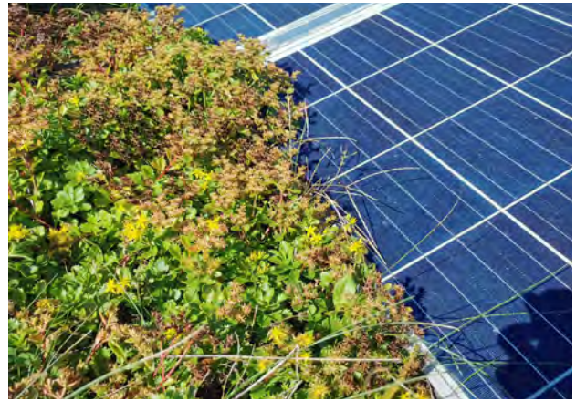
Insufficient spacing Credit: Weiss-Tessbach
