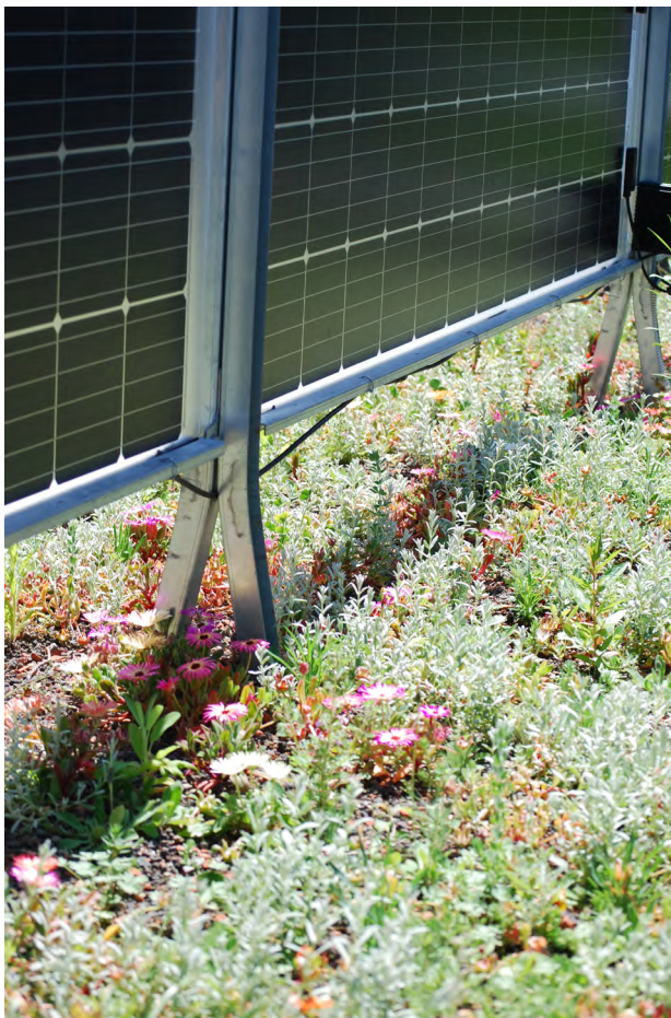
Bifacial panels on a green roof, Switzerland
