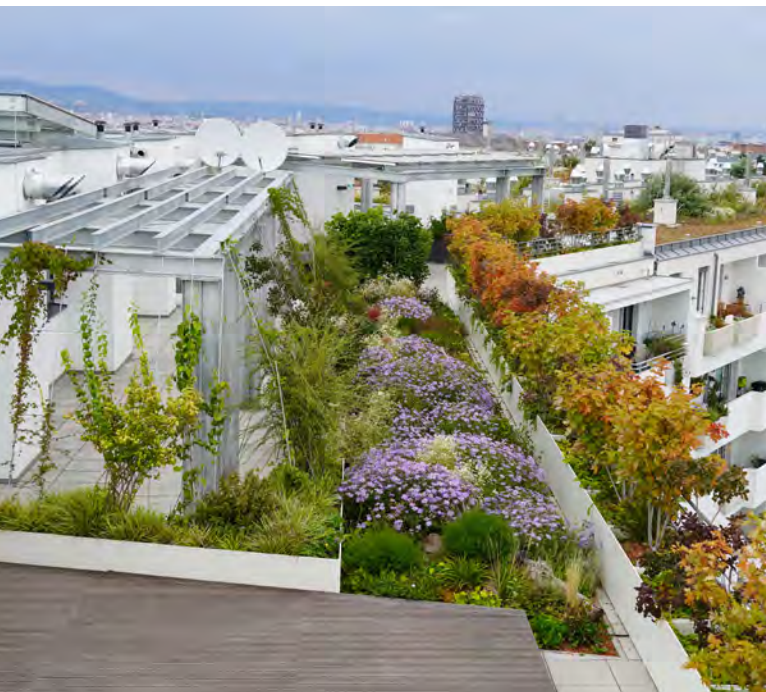
PV roof garden on a residential building Biotope City Wienerberg, Vienna Credit: Irene Zluwa
