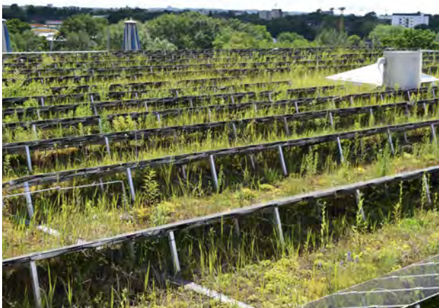
Before maintenance. Credit: BuGG
