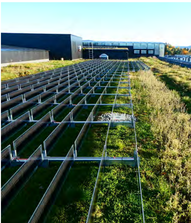
Vertical Bifacial Panels on an Oslo office building
