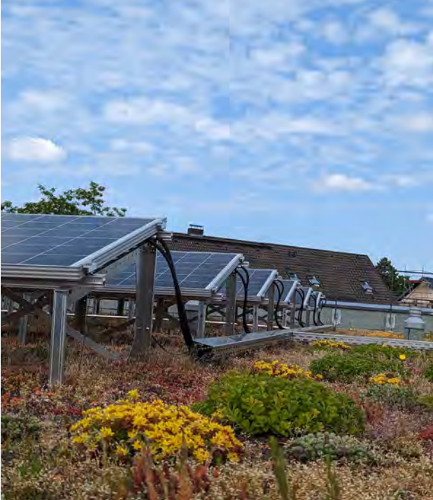
Solar green roof on a kindergarten in Dresden Credit: BuGG
