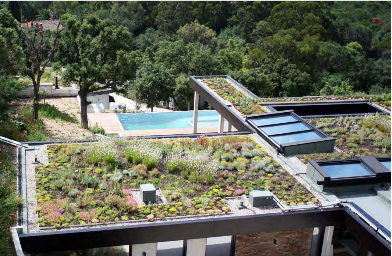
Green roof on a private house in the South of France, aiming to provide cooling in summer Credit: Biotopes Creation
