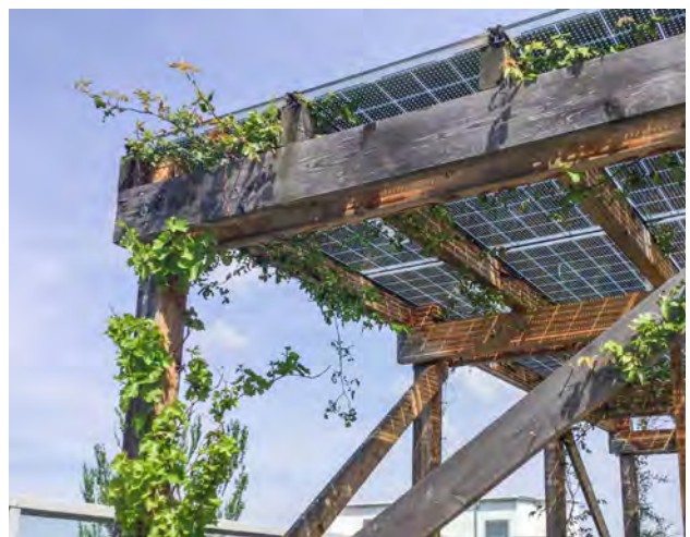
PV roof garden
