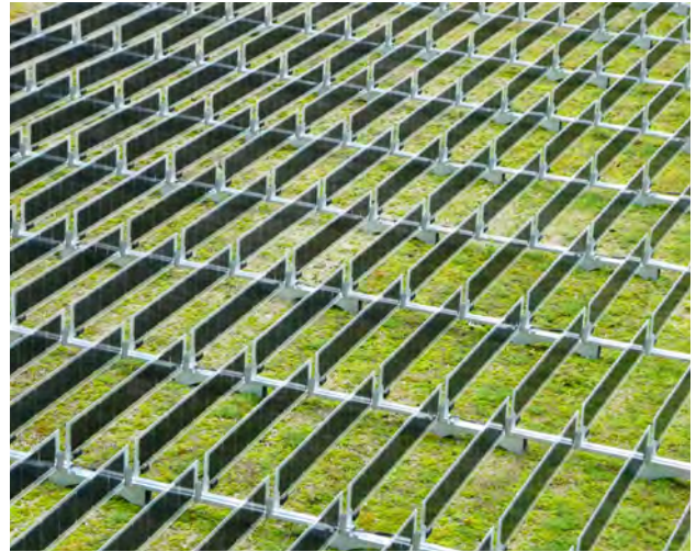
Vertical Bifacial Panels on an Oslo school building Credit: Over Easy Solar
