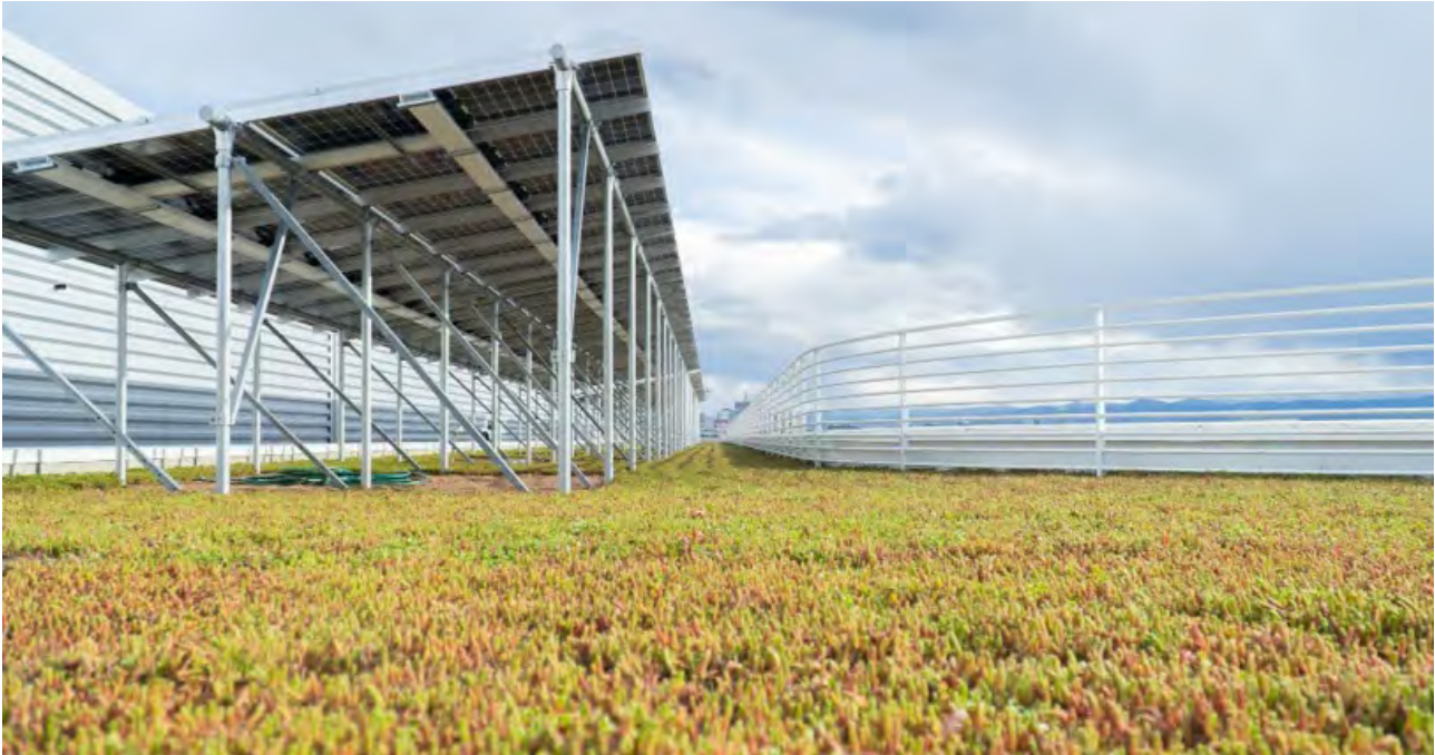
Green roof beneath solar PV array
