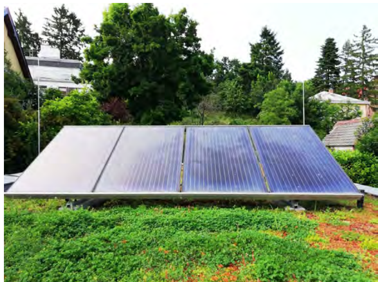
Hybrid PVT collectors on a green roof Credit: Alexander Friedrich
