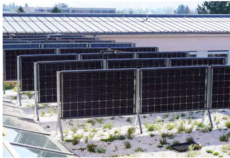
Project GREENsChOOLENERGY - Testing innovative combinations of solar/greening combinations for cooling buildings and outdoor spaces - Klagenfurt, Austria Credit: Irene Zluwa, GrünStattGrau
