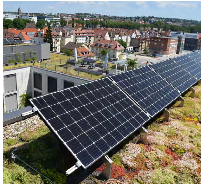
Solar green roof, Germany Credit: BuGG
