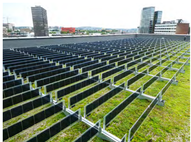
Vertical Bifacial Panels on an Oslo school building Credit: Over Easy Solar
