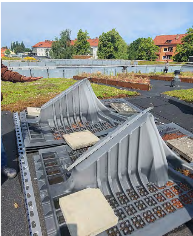
Integrated Ballast Credit: Steven Peck
