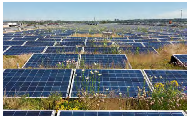
Overgrown PV modules due to insufficient spacing Credit: Elisabeth Weiss-Tessbach
