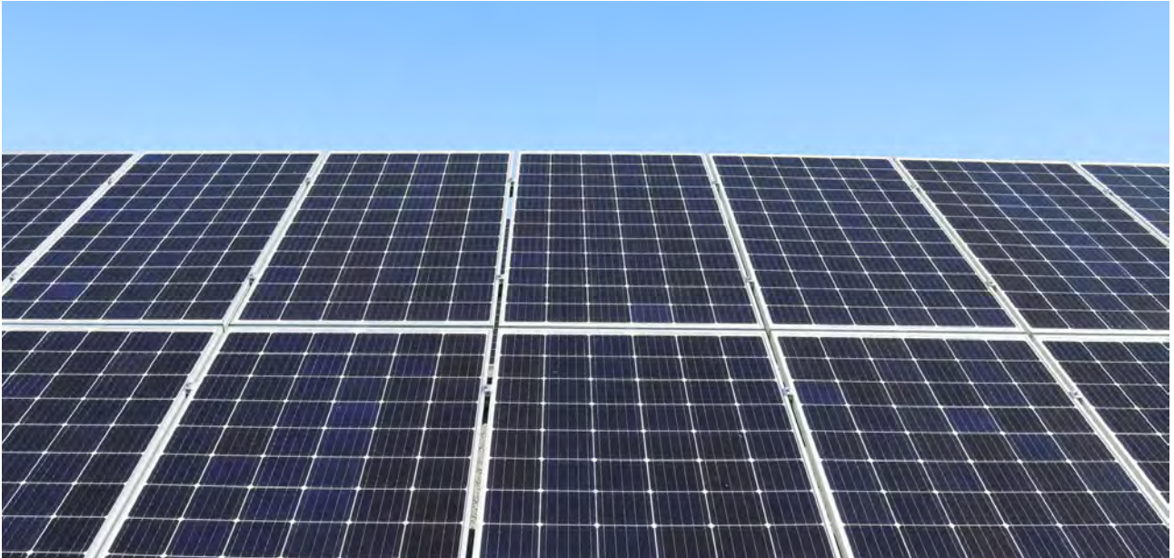
Monocrystalline solar panel array Credit: CEC - Lee County Electric Cooperative
