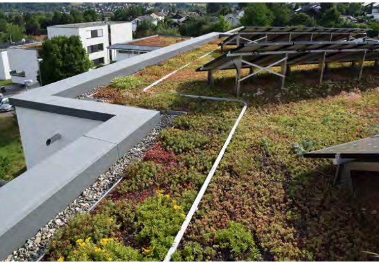
Integration of fall protection into the solar green roof system on a roof in Nürtingen
