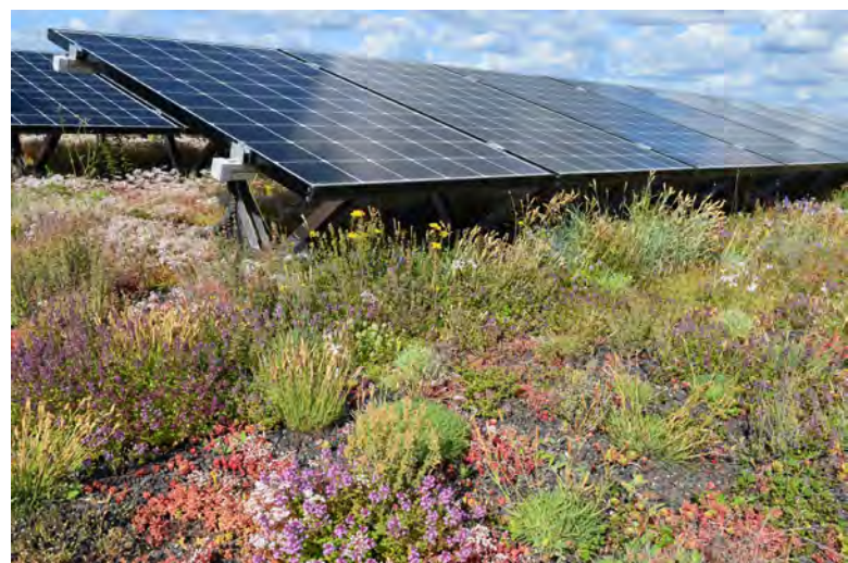
Solar green roof in Stuttgart Credit: BuGG
