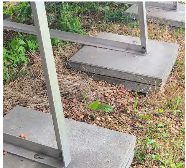
Non-Integrated Ballast Credit: Steven Peck
